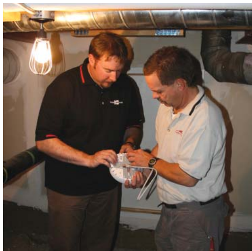
Once installed, the D-Link wireless APs can now be controlled remotely from one centralized server room.
