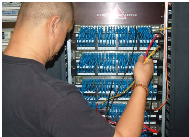
Tornillo Independent School District IT Support, Sergio Sosa, installing the D-Link xStack switches and uplink modules, which helped provide the district with a solid, reliable 10Gigabit network.
